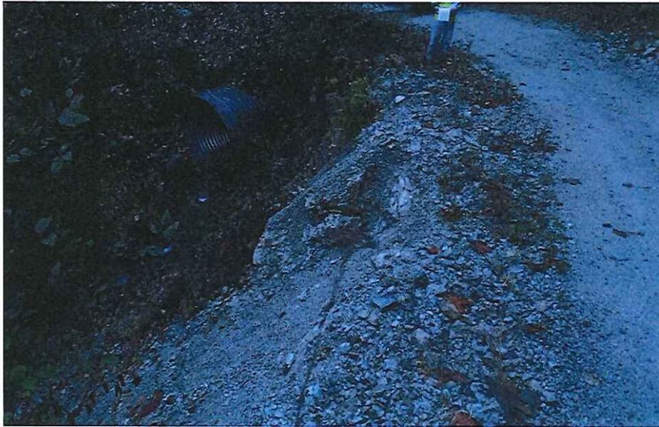
CK2211 Right Approach Fill erosion
